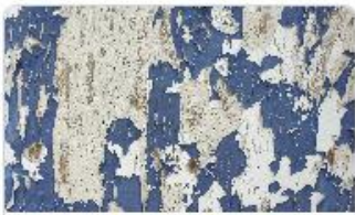
Defects in Modern Building
